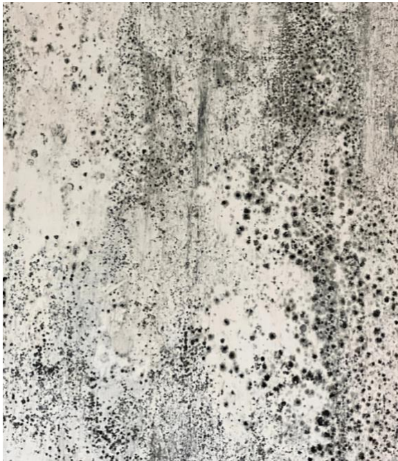
Figure 10: Old wall with mould stains background
