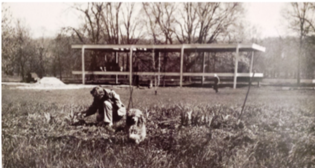
Figure 140. Dr. Farnsworth with her dog, her house under construction ca. 1949. View of the north face of the house showing the structure which differs little from the end result. National Trust for Historic Preservation archive.
