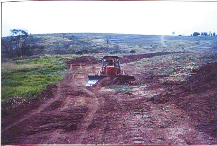
Figure 85: Unpaved road maintenance on sugar cane plantations. © UDOP
