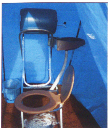
Figure 72: Sanitary canvas as an example of improvised toilets on plantations.
