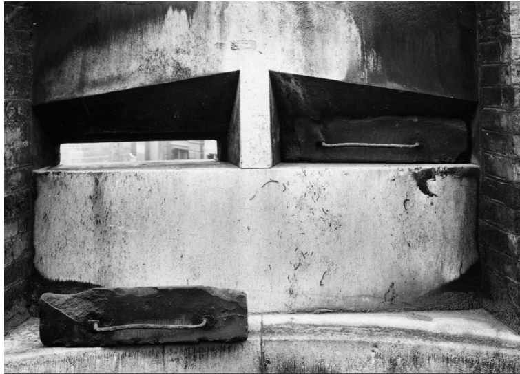
Fig. 16: The Bank of England, Threadneedle Street, City of London: the bullion yard showing detail of the stone defences , Joel Humphrey (1930), black and white photograph. (RIBA92157)
