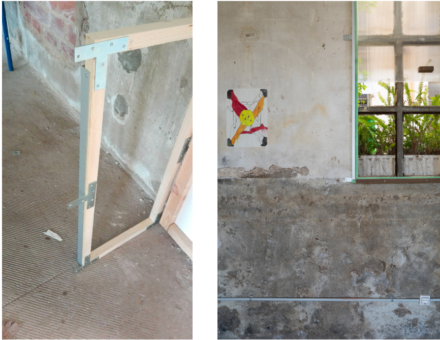
Window mock-up (left) and details (middle and right), photos by Gabriele Basilico.
