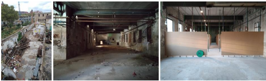
Figure V-20. Left: Warehouse Foseco in la Escocesa industrial complex collapsed in less than a decade due to deterioration derived from unuse, despite an architectural competition was held and the project ready to be built. Middle: Warehouse L of la Escocesa as found in 2019. Right: Warehouse L in 2020 ready for artists to occupy the workshops.
