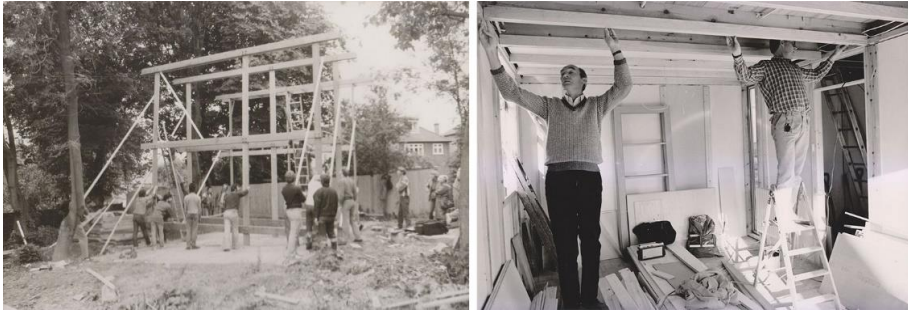
Figure III-15. Walter Segal developed a construction method based on easily available timber frame construction that allowed residents to design their own houses. Segal was in charge of supervising the works. This was famously put in practice in Lewisham, London, during the 1970s. There are over 200 houses built using the Segal method in the UK. Source: ribaj.com, M. Charles, J. Broome (pictures) and Broome, 1986 (sketch).
