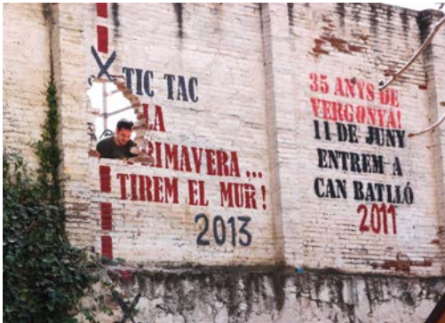
Demolition of the wall by neighbours with a painting of "Tic Tac can Batlló".
