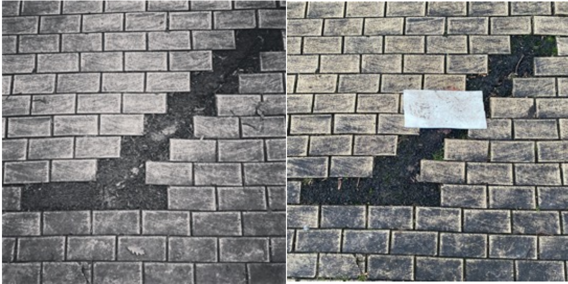
Figure 44. Ten missing bricks, London (2020) © 2020 Alison Rees. All Rights Reserved.
