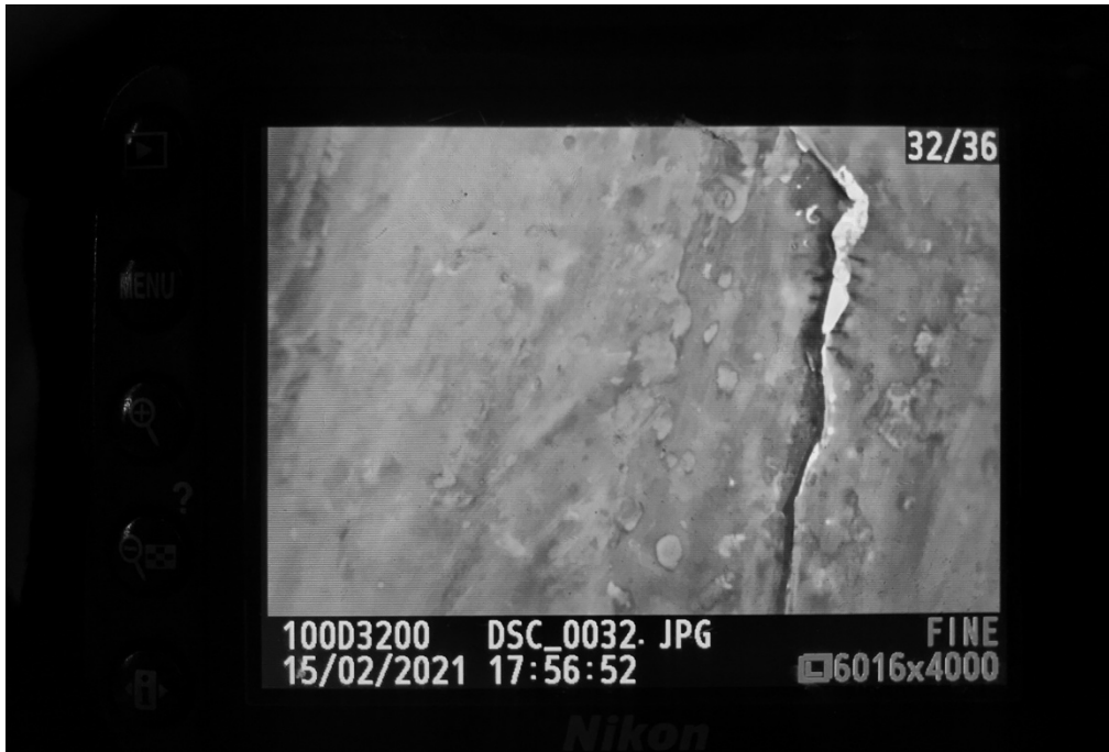
Figure 16 Photograph of the Crack. Kyriaki Spanou.
