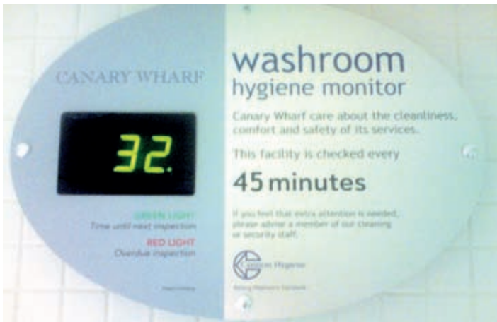
This countdown clock reassures people that the toilet is regularly visited, clean and well managed.
