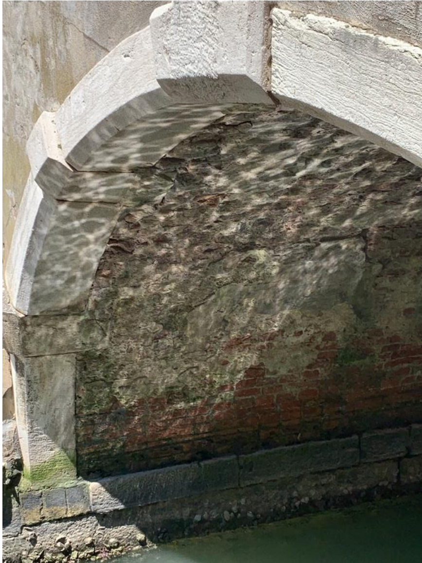
Figure 25 Example of a flickering image under a bridge
