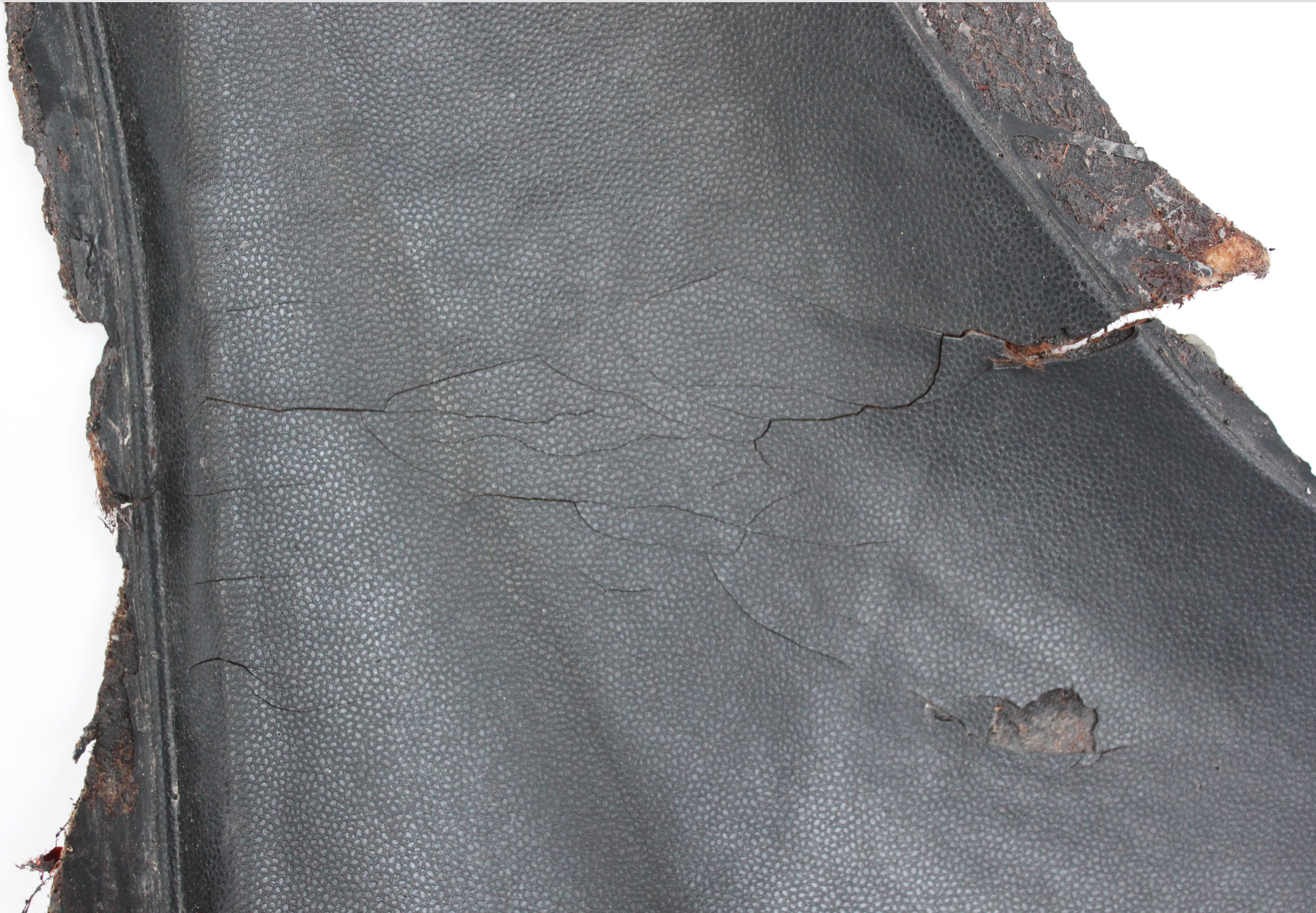
Detail showing flaws in the bio-resin surface in the broken part of outer door panel
