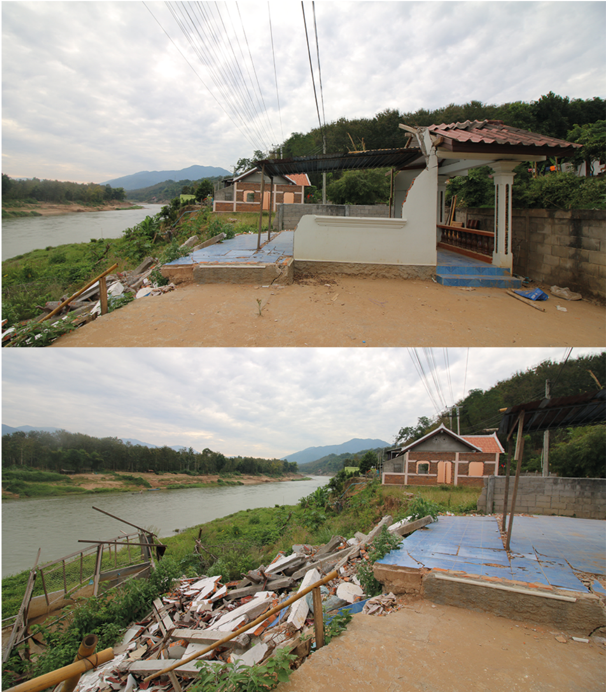
Figure 18.b Examples of a house collapsed by flooding. Photo by Soon Min Hong.
