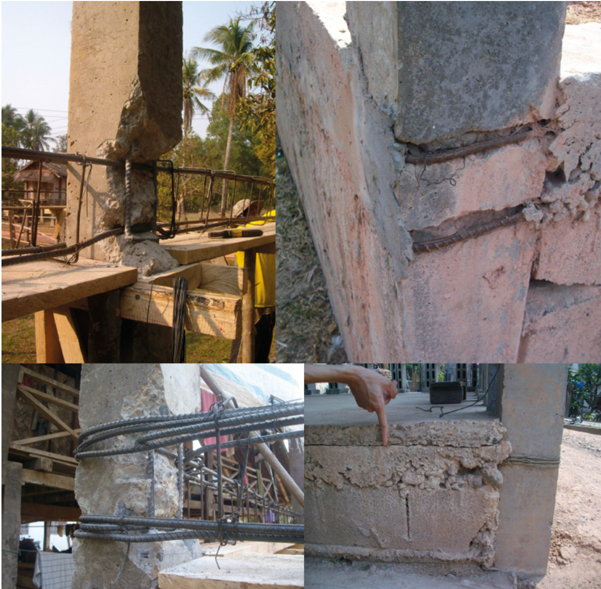
Figure 28. Examples of construction failure and damaged building elements. From Guidelines on Housing Construction in Disaster Prone Areas (2014).
