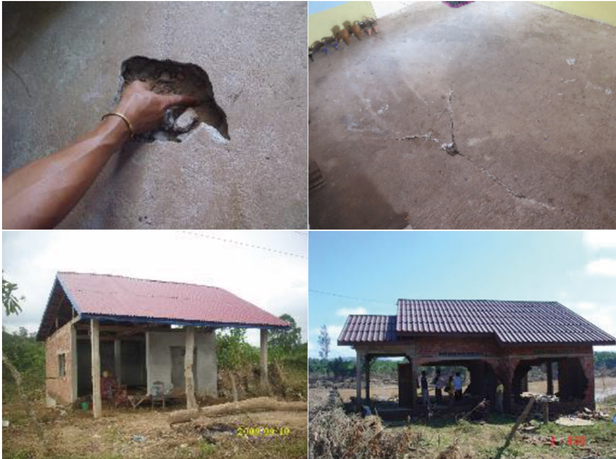
Figure 18.a Examples of housing elements damaged by flooding. From Guidelines on Housing Construction in Disaster Prone Areas (2014).
