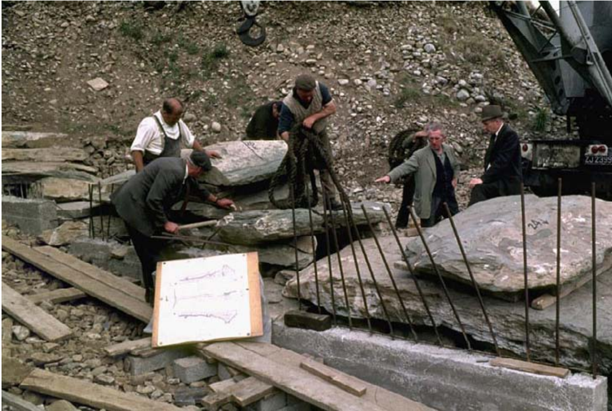
Figure 95a Michael O'Kelly (second from right) during reconstruction work at Newgrange, early 1970s. Reproduced in Geraldine Stout and Michael Stout, Newgrange . (Cork: Cork University Press, 2008), 47.
