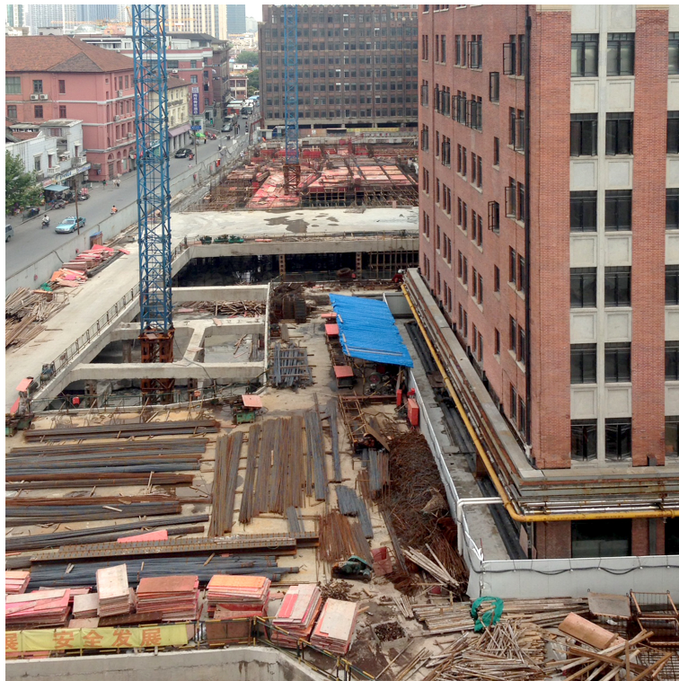
Figure 72: Ongoing construction work to deliver Phase 2 of the masterplan (photographed by the author)
