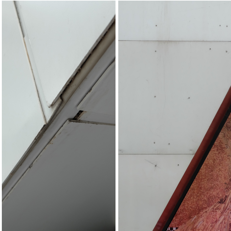
Figure 53: (Far left) Poor construction detail and finish at Zaha Hadid's Galaxy Soho, in Beijing (photographed by the author)
