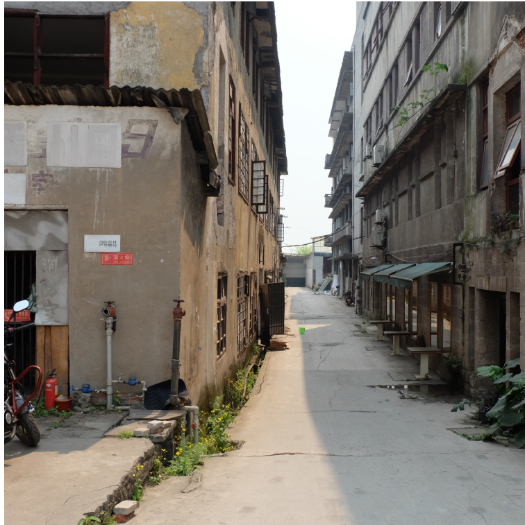
Figure 57: The condition of the existing ex-industrial buildings in Eling that formed the Testbed II site (photographed by the author)
