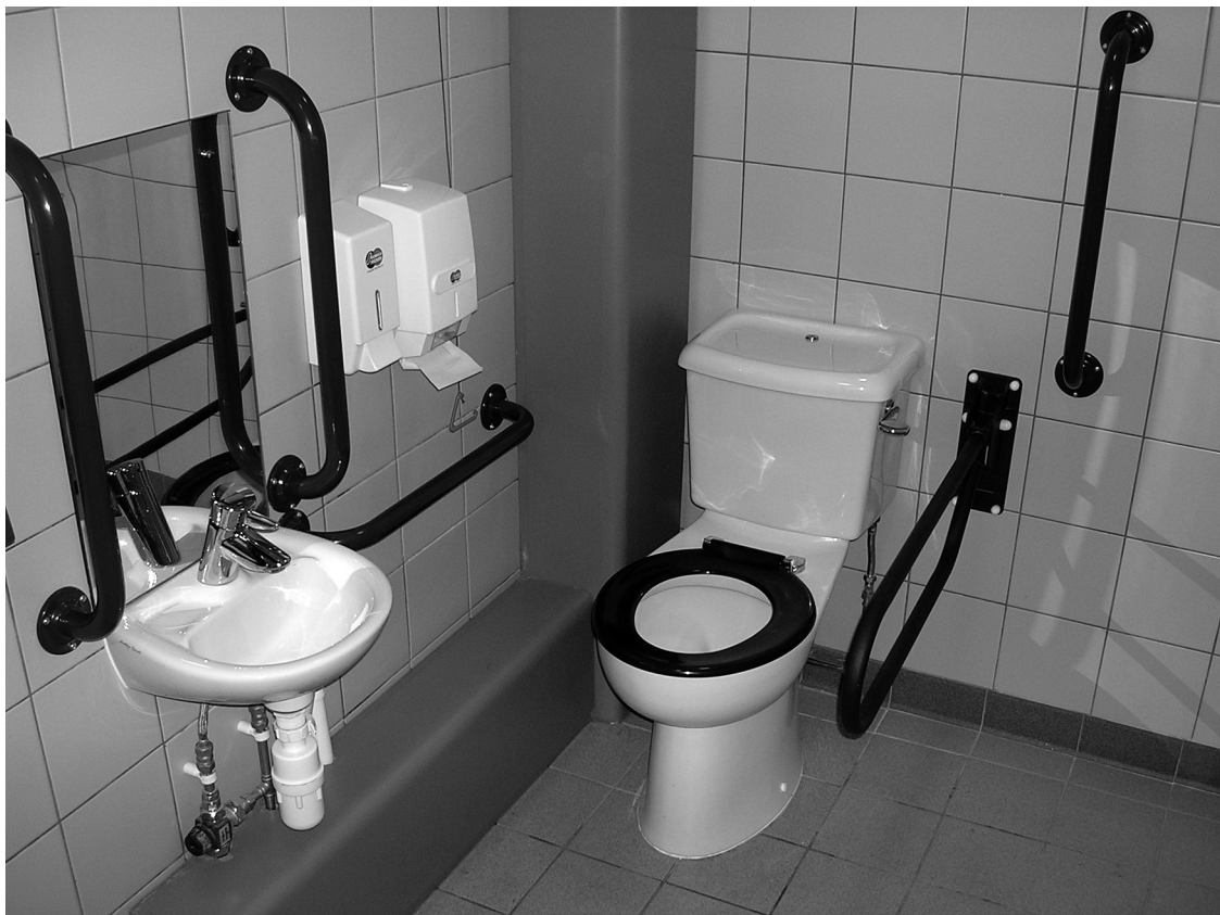
Figure 4. The unisex accessible cubicle (note alarm is incorrectly installed). (Source: Bichard, 2006)
