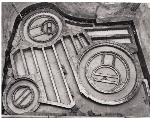
Fig.40: Tesoro di San Lorenzo, Genoa, 1952–6, aerial view of the museum's foundations, exhibition design by Franco Albini and Franca Helg.
