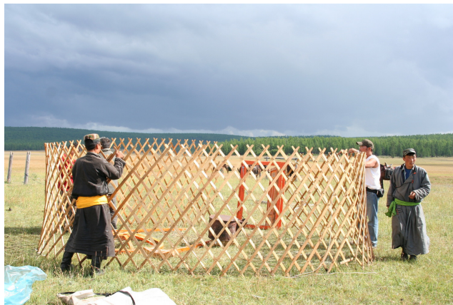
Figure 4.10: First stage of setting up a ger: unfolding the lattice structure. “Montage d’une Yourte” 2007, Mongolia, photo by: Alix Guillard (Wikipedia [no date] c)
