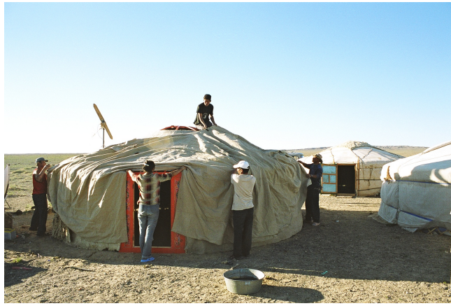
Figure 4.12: Mongolian ger: adding the outer cover, the inner cover can be seen underneath, the gers in the background are complete. (Wikipedia [no date] c)
