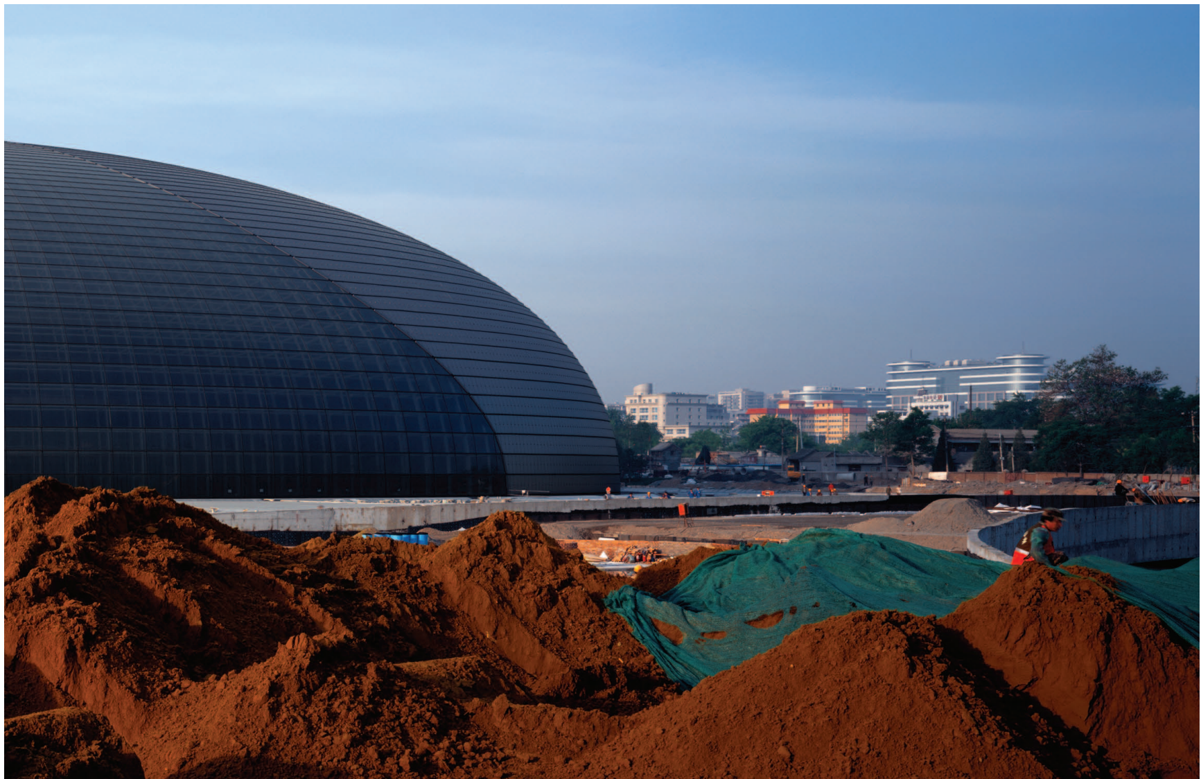
Drop Down Sculpture The new Beijing Opera by French architect Paul Andreu under construction in 2007
